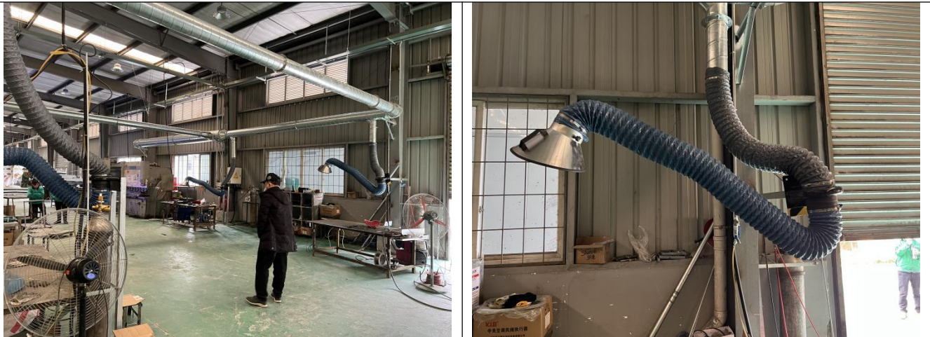
焊接工位焊烟集气罩
